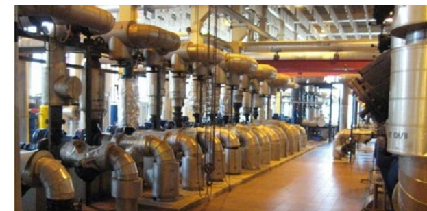
Air-Cooled Chilled Water Plant King Faisal Specialist Hospital, Riyadh, Saudi Arabia
